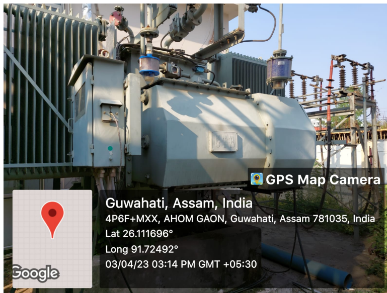
Wheeling to the Grid
